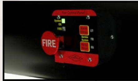
SMVS Control Panel
